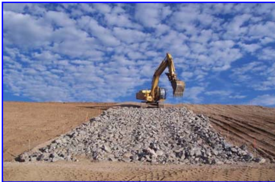
This trackhoe is placing rip rap on the interior of the dam face to help prevent erosion of the banks.
